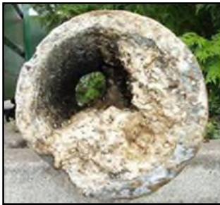
Grease clog in sewer pipe.
